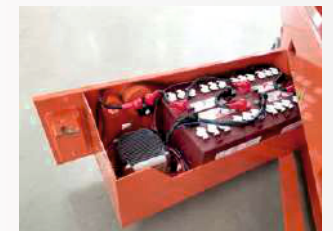
Trojan Battery Pack And Charger
